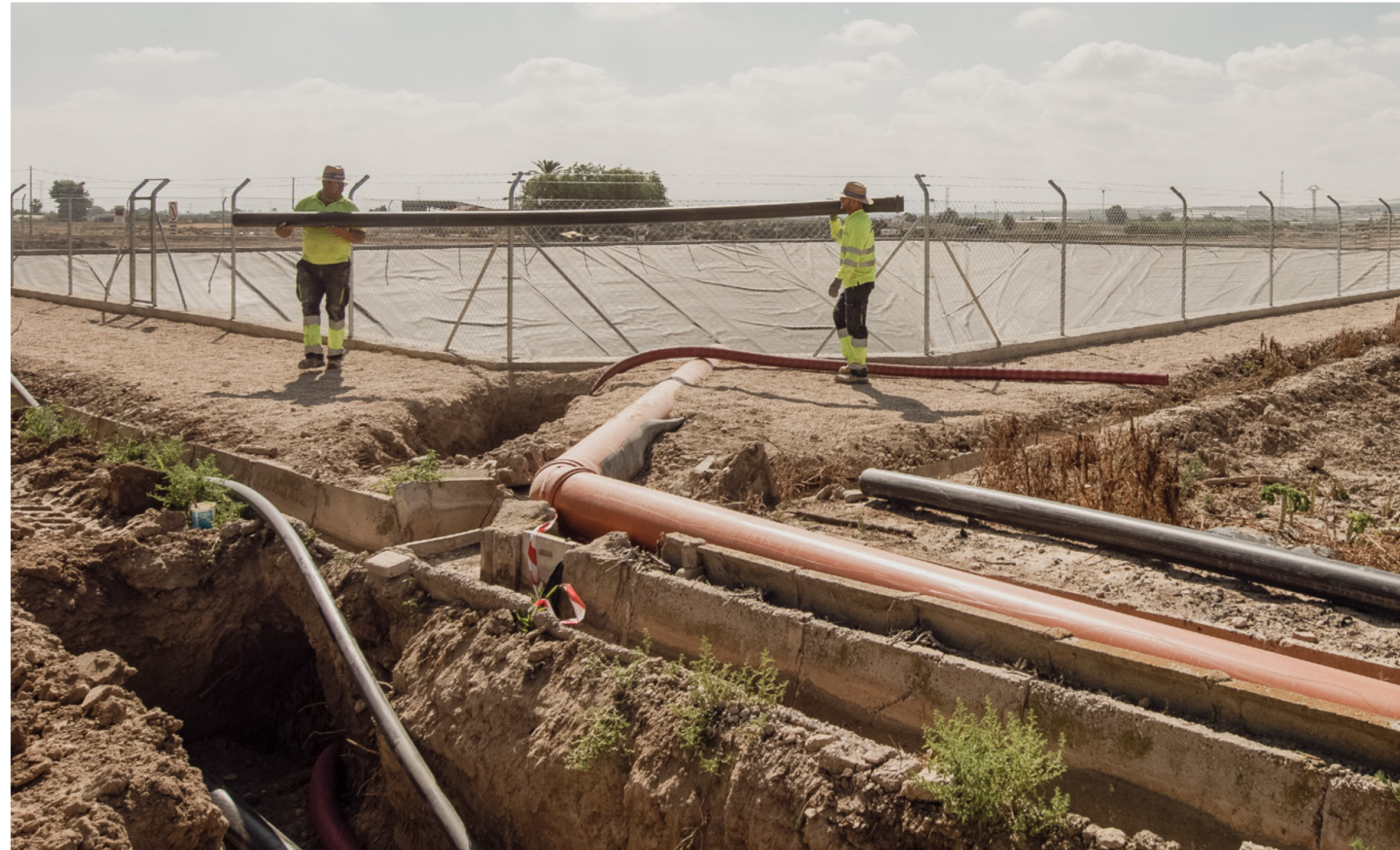
Operators installing a drip irrigation system next to an agricultural reservoir in the area of Lorca, Murcia. ©González-Cebrían
