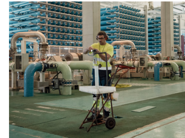
Alicante desalination plant. ©González-Cebrián
