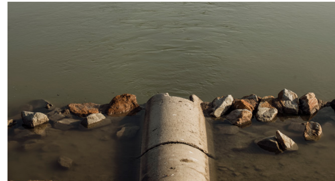
Water pipe in the Mar Menor salt flats, Murcia. ©González-Cebrián
